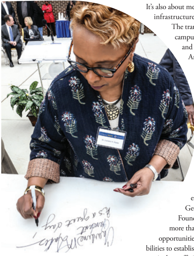
Dr. Charlene M. Dukes leaves an indelible mark on the last beam placed in the Queen Anne Building.
